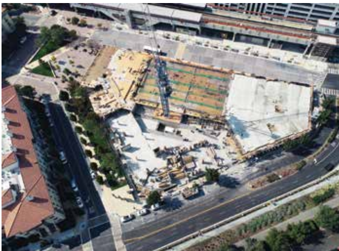
Fig. 1: The project site comprised a ground-level slab (lower left) and a podium level (right) (photo courtesy of BKF Engineers)
